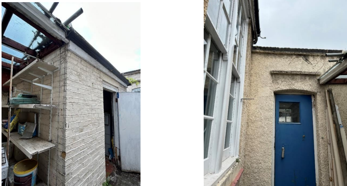
Figure 11 – Example condition of existing ad-hoc extensions
